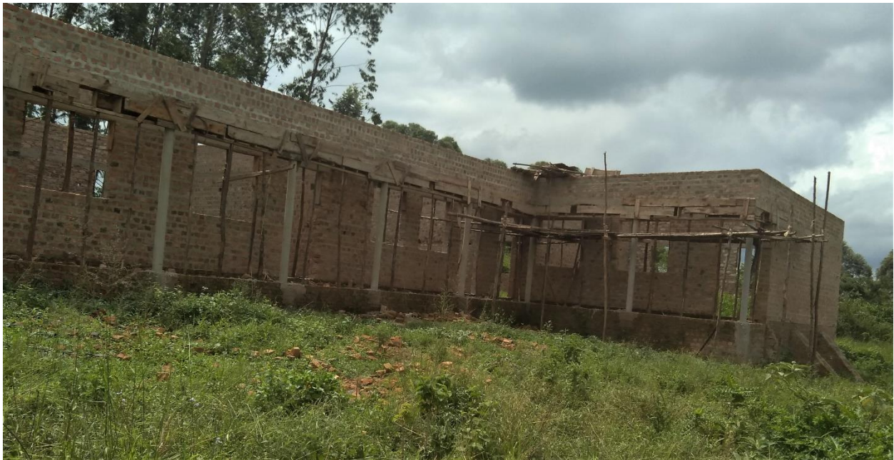
Current structure under construction at St. John Paul II vocational secondary school at Mityana
